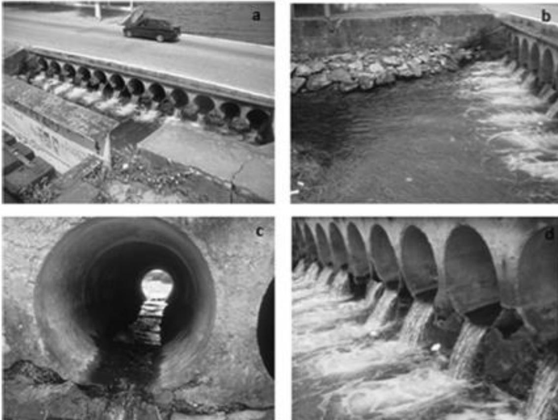
Fig. 3. Underneath culverts from bridges built in Doce River (for bridges' location see Fig. 1).
